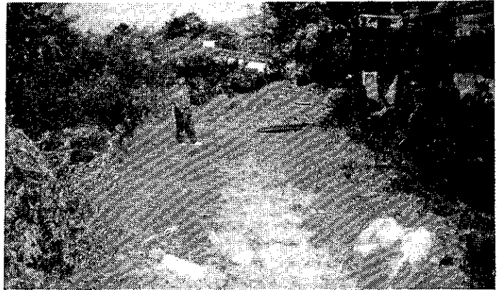
FRUITS OF WRATH: Mr Leonard Meyer's orchard was dug up to lay a pipe without his consent
