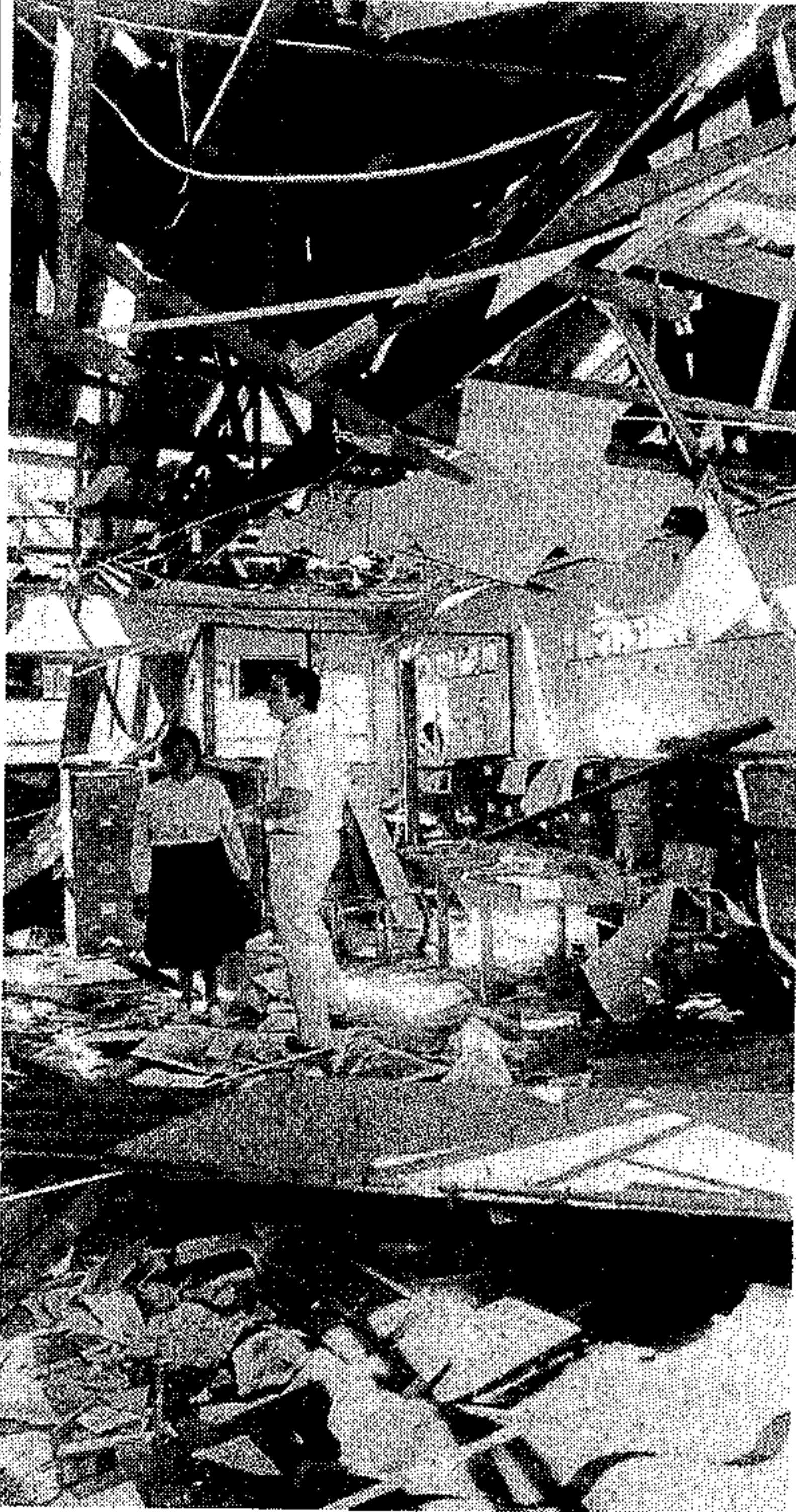
Damage caused to the Kwa Mashu township offices when two blasts rocked the building late Monday night.
